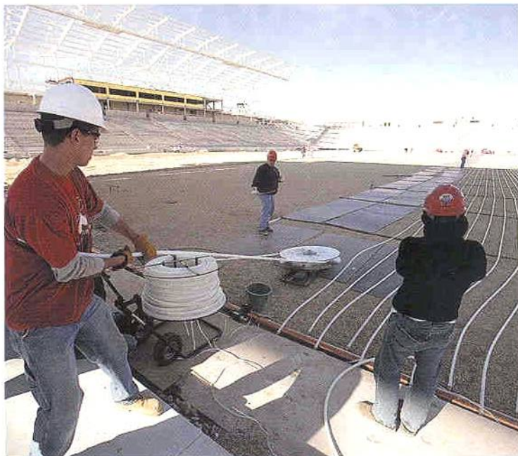
Motorized sled, custom-made for the project by Althoff Industries, carried the loops of PEX tubing from one end of the playing field to the other.
